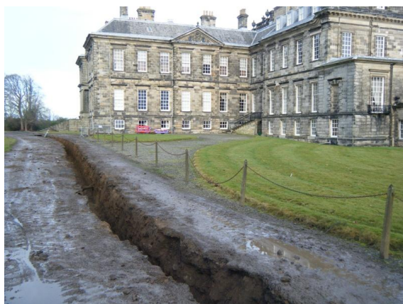
Illus 2: View of Trench 2 to the rear of Hopetoun House, facing north
