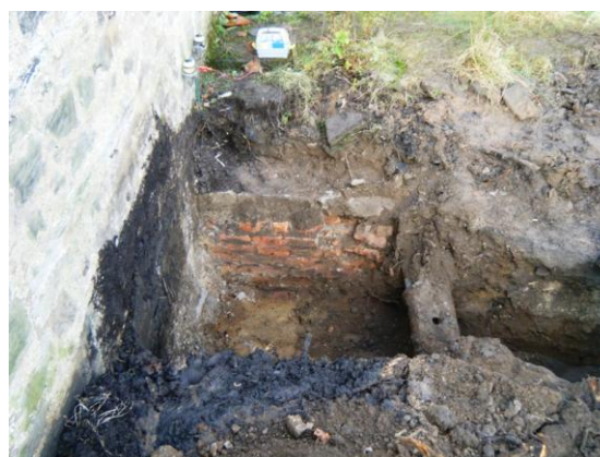
Illus 9: View of south facing section at the north end of Trench 5 showing culvert 021.
