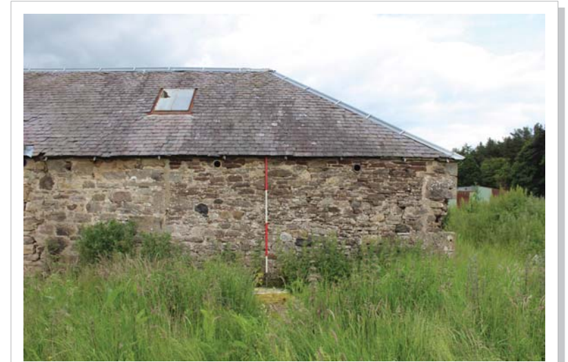
ILLUS 12D West range, west elevation, detail of different construction at south end (070)
