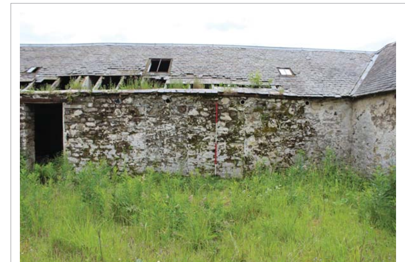
ILLUS 13C South range, north elevation, detail of blocked doors to west of G14 (046)
