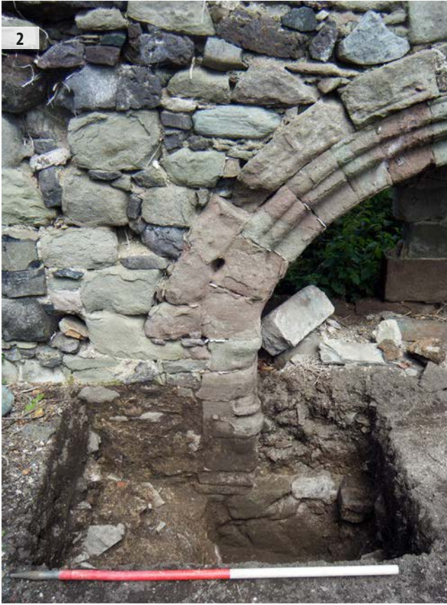
ILLUS 2 Wall face and lower part of recess exposed in Test Pit 1. From S
