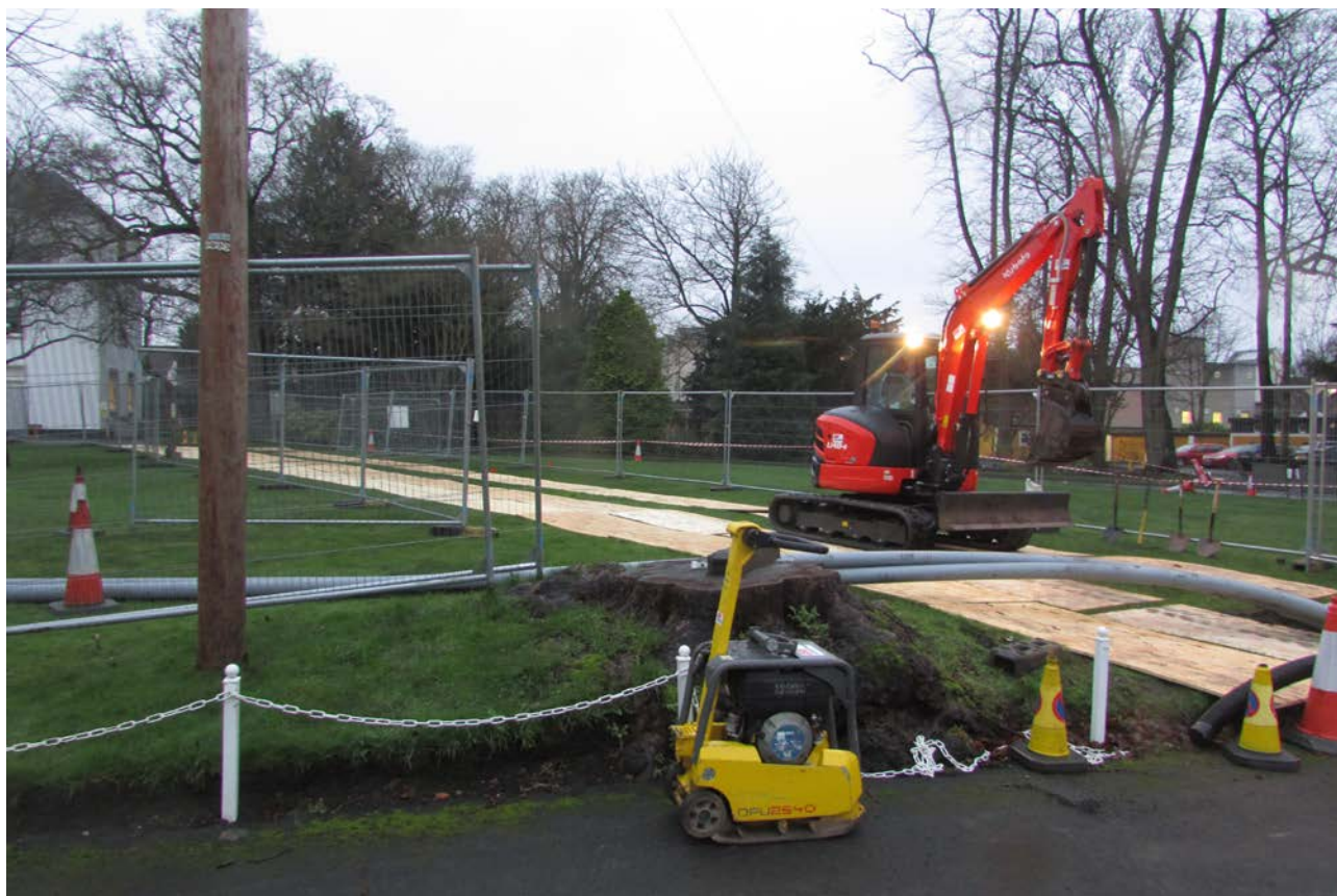
ILLUS 2 Site overview showing cable route set out in between plywood boards
