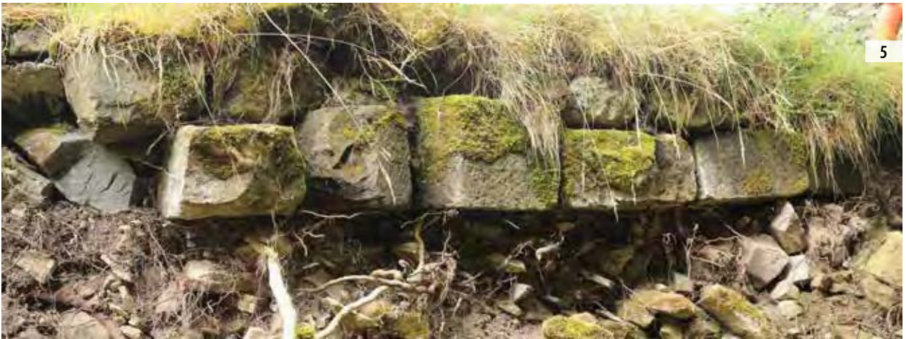
ILLUS 4 W facing view of cemetery wall ILLUS 5 W facing view of eroded bank with faced stones
