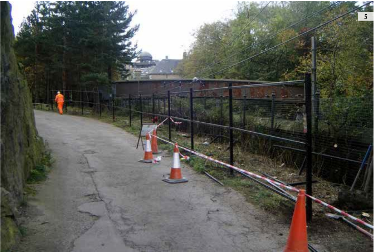
ILLUS 3 Manual excavation of the holes ILLUS 4 Excavation of hole under the Middle Footbridge ILLUS 5 General view of the fencing line east of West Footbridge, facing west
