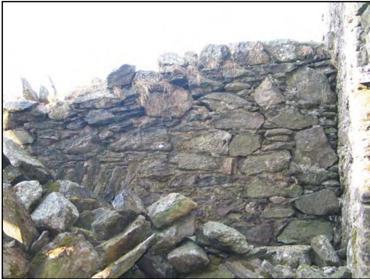
Plate 23 - Interior, SE block, collapse and blocked fireplace in SW gable
