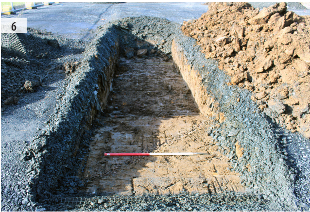
ILLUS 4 East facing section of Trench 1 ILLUS 5 View of linear cut [3002] in Trench 3 ILLUS 6 View of drain in Trench 4
