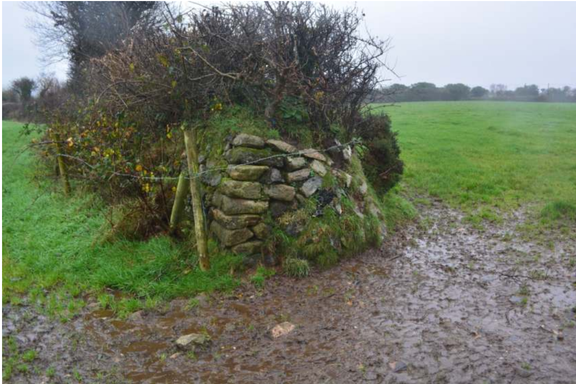
Plate 9: Partial stone wall and hedgerow in northern area of PDA/Area 1 (HA1), looking north
