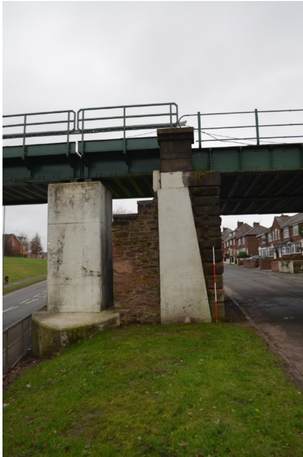
Illus 24. Detail of Illus 23 showing the former line of the embankment retaining wall.
