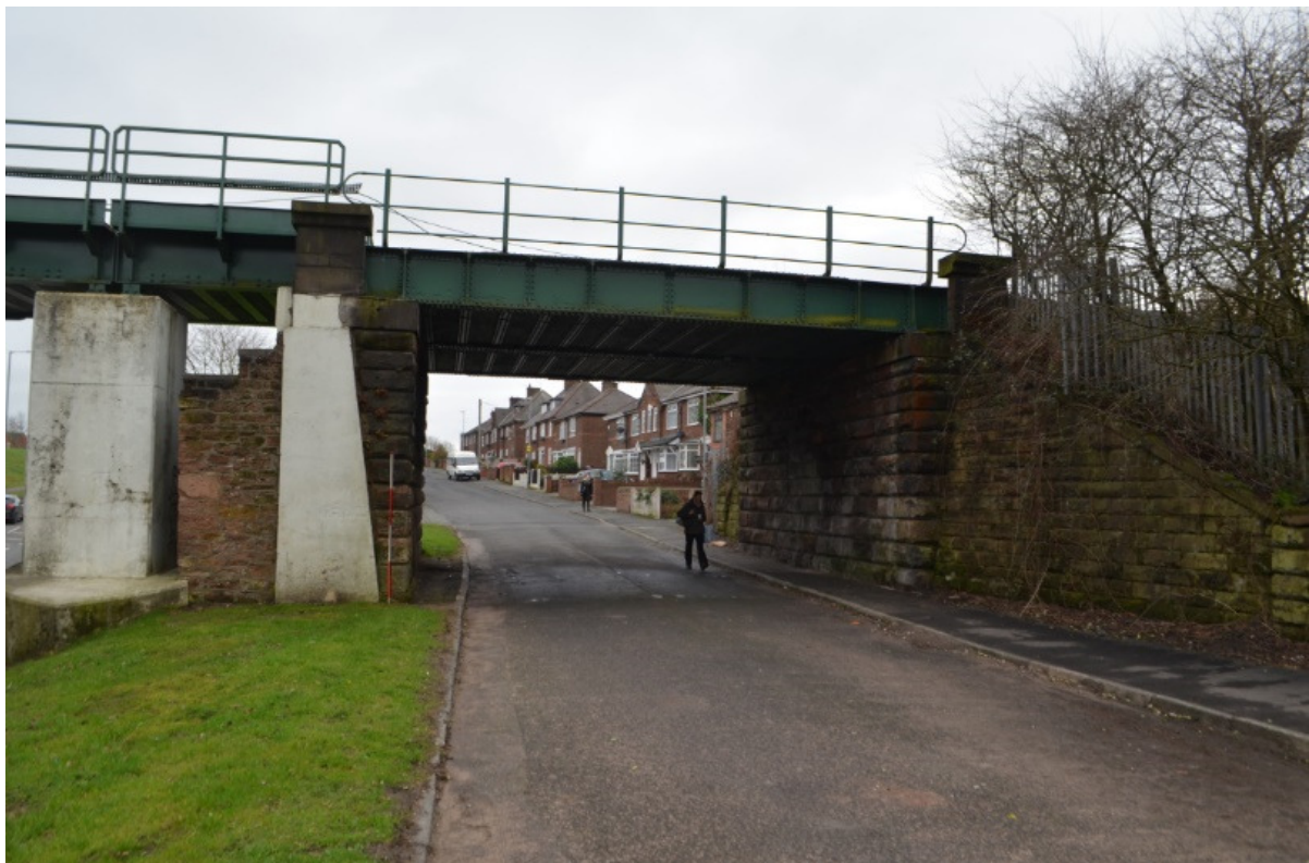
Illus 23. Detail of the northern side of Underbridge 55 showing Phase 1 piers and retaining wall and Phase 2 trackbed. The former line of the eastern embankment retaining wall is defined by the white painted concrete.
