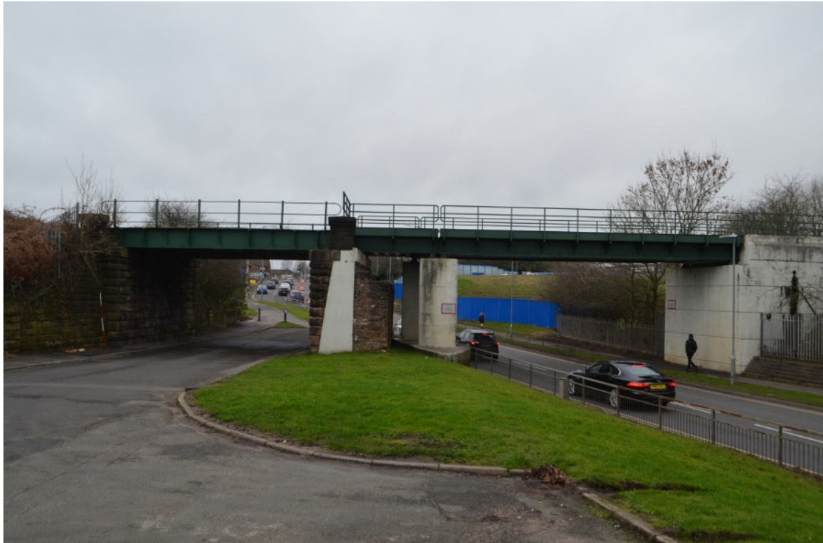
Illus 20. View of Underbridge 55 from the south. The original line of County Road is on the west (left).
