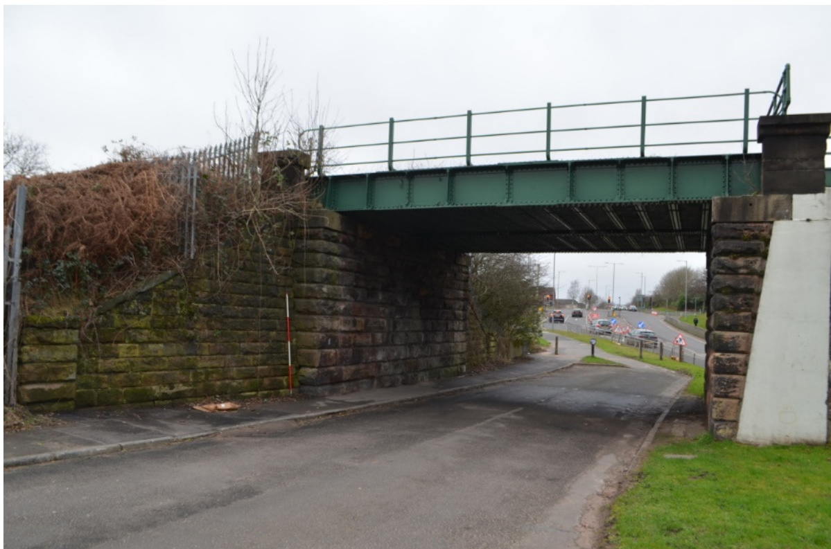
Illus 21. Detail of the southern side of Underbridge 55 showing Phase 1 piers and retaining wall and Phase 2 trackbed.
