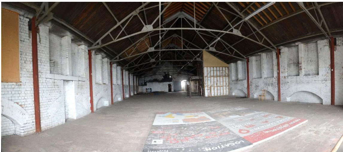
Illus. 76. Panorama of Room FIF.1 from its eastern end, looking south-west to north-west
