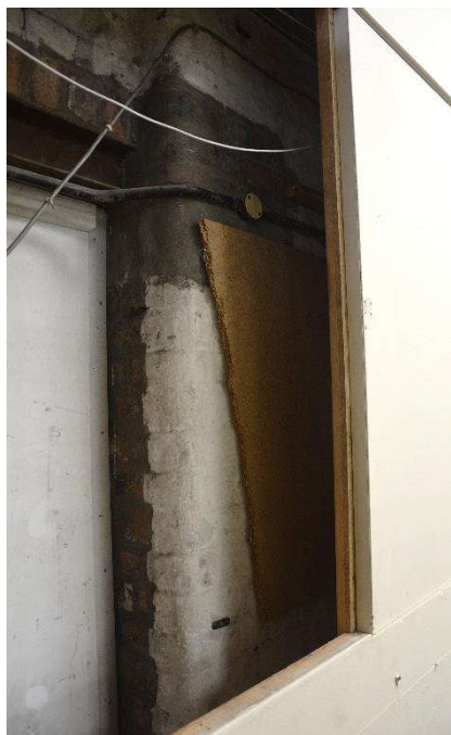
Illus. 43 (above). Historic fabric behind stud walling on staircase between Room FST. 6 and FSTM.3, looking south-west
