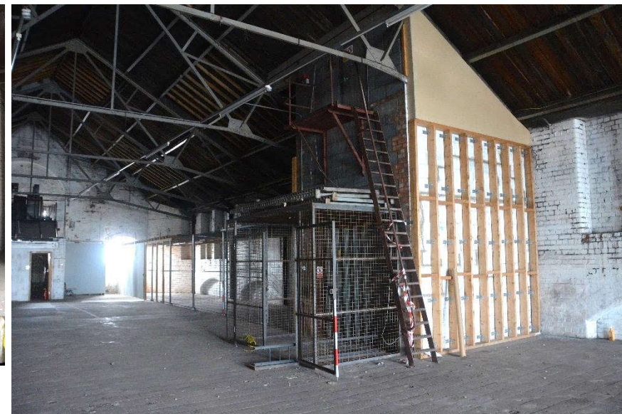
Illus. 77. Metal storage area for Gardiner Haskins in north-west corner of Room FIF. 1 and lift
