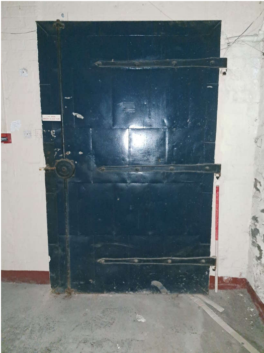
Plate 205: Metal door in the northern end of the western elevation of Building 5. 1 x 1m scale.
