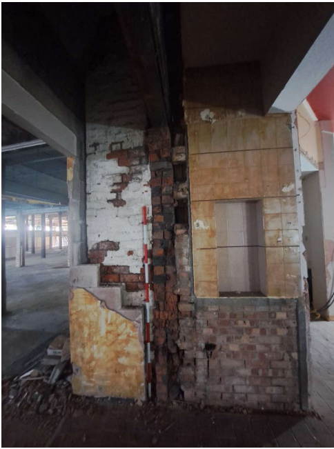
Plate 190: Detail of opening in elevation between Buildings 2 and 4 on the first floor. At the left the 1880s build of Building 4 can be seen, with early 20th century addition in the middle and post-1958 addition on the right. 1 x 2m scale
