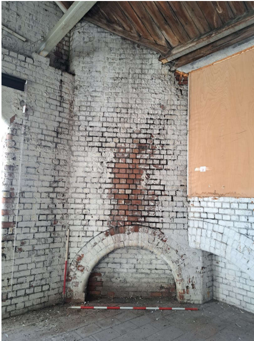
Plate 182: Detail of the chimney in the south-east corner of room FIF. 1 (Building 1). 1 x 2m scale, 1 x 1m scale
