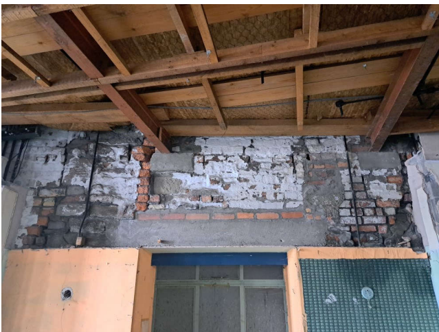
Plate 196: Detail of blocked opening in the north-west wall in Building 3. Also the southern elevation of Building 4. Shows a mix of brick and stone and may indicate remains of Phase 1 soapworks buildings incorporated into the 1880s (Phase 2) southern elevation of Building 4.
