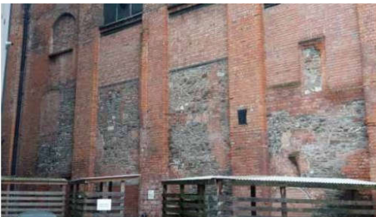
Plate 176: Areas of pennant stone in the southern elevation of Building 1. No scale
