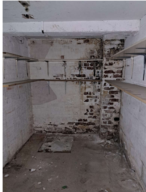
Plate 199: Area of Phase 2 brickwork visible in the northern wall of Building 4. No scale
