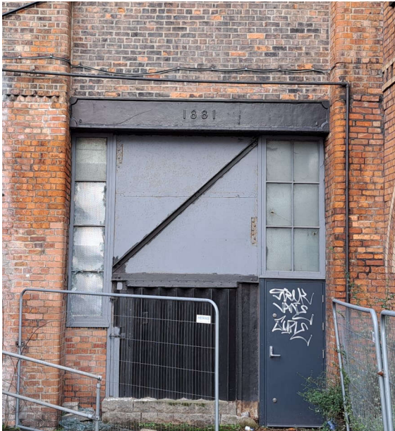
Plate 174: Detail view of doorway in western elevation of Building 1. Shows date of '1881' with initials C and J on opposing lower corners. No scale.
