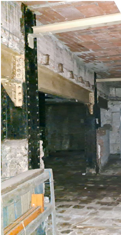
Plate 194: Looking north-east along wall between basement rooms B.1 and B.2. Cut off I-beams can be seen as well as larger stanchions forming the wall. No scale
