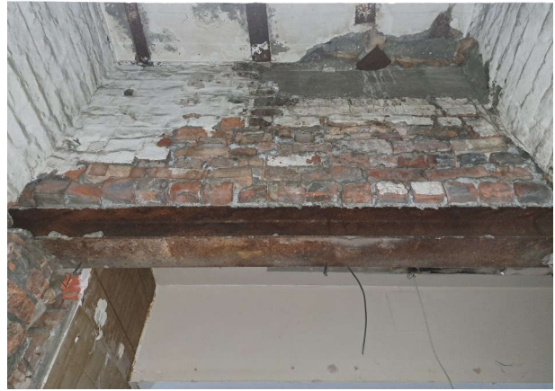
Plate 191: Detail of 1880s (Phase 2) brickwork of Building 4 with Phase 3 steel lintel below. Taken looking west in opening between Buildings 2 and 4 on the first floor. No scale
