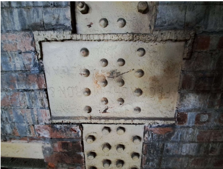
Plate 191: Detail of stanchion plate forming the wall between Buildings 2 and 3. Inscribed 'Frodingham Iron &... England'. No scale
