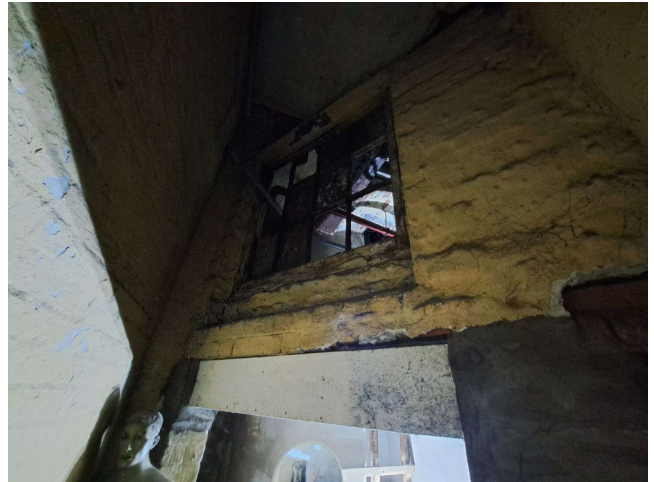
Plate 187: Early 20th century window in eastern elevation of the lower ground floor stairwell (LG.2). The wall to the left is a later addition and the window once provided light to room LG.1 No scale.
