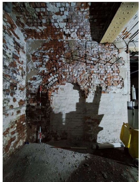
Plate 177: Detail of double arch feature on northern elevation of room LG 1. 1 X 2m scale, 1 x 1m scale.
