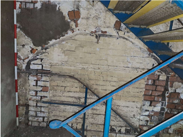
Plate 186: Blocked window in western elevation taken from lobby between lower ground floor (LG 2) and first floor (FIR.2) of Building 1. Shows several phases of blocking. 1 x 2m scale.
