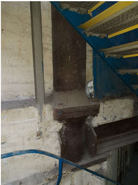
Plate 188: Detail of internal steel frame of Building 1 taken from lobby between lower ground floor (LG 2) and first floor (FIR.2) of Building 1. No scale
