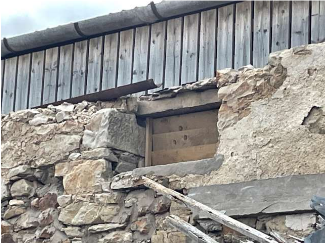
Detail of remains of a window on the north elevation of Building 1
