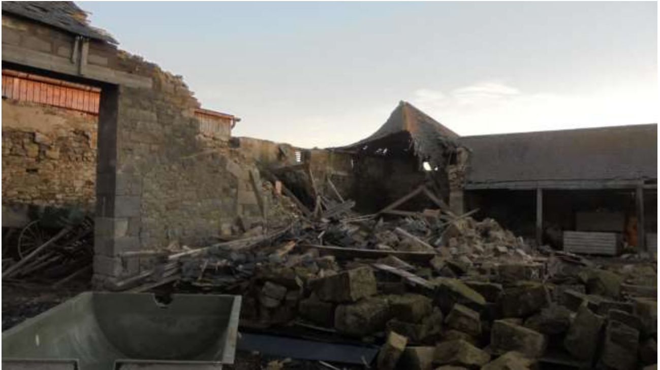
Detail of damage to south elevation of Building 1
