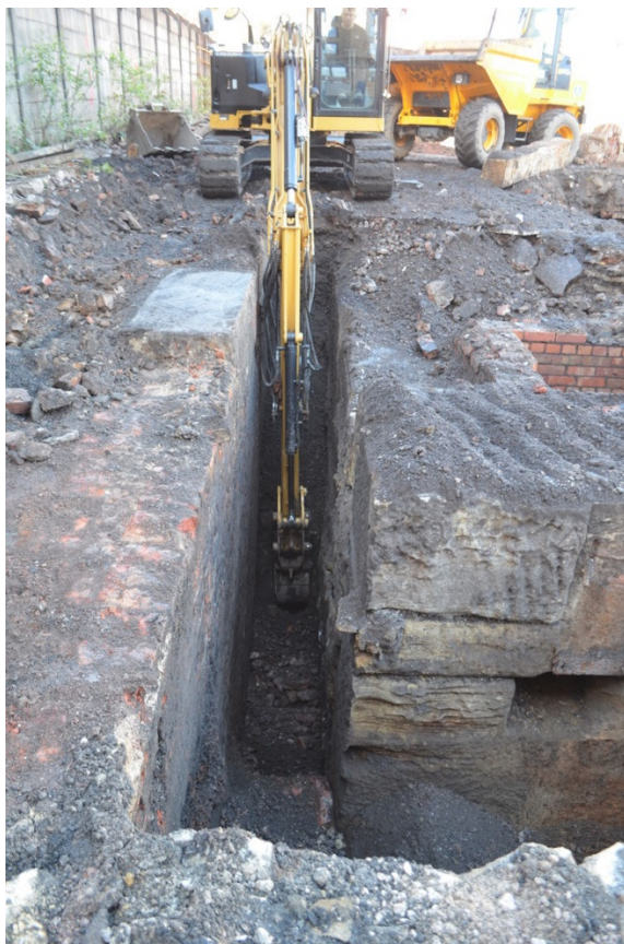
Illus 29. Excavating the flywheel pit on the eastern side of the Engine House. View looking north.
