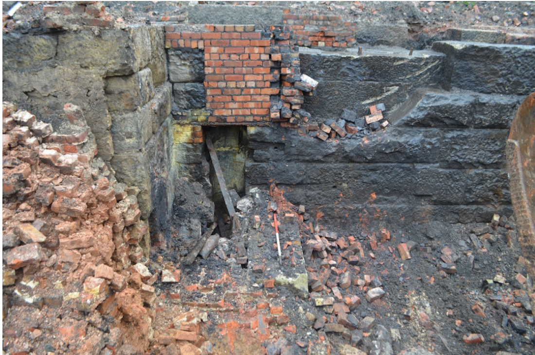
Illus 28. The Engine House during demolition showing the recesses for a water pump and flywheel gear exposed in wall [94]. The brickwork in the centre of the view is for a 20 th century inspection chamber. View looking west, scale 1 m.
