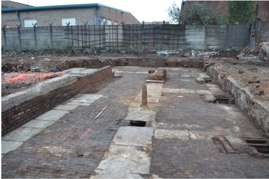
Illus 38. The factory extension looking east, a cast-iron pillar found in the demolition fill has been placed in the socket on stanchion [100]. View looking west, scales 1 m.
