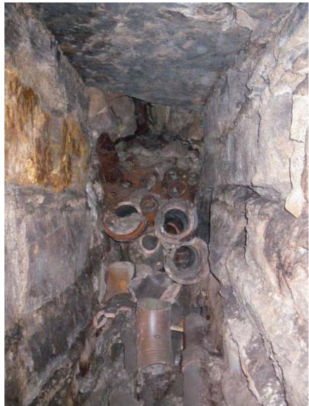
Illus 21 Blocking of culvert structure 6
