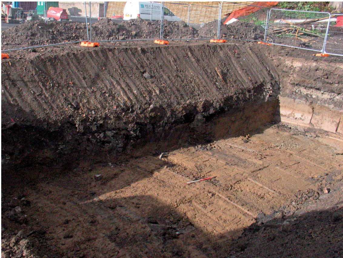
Illus 4 View of the fuel tank trench showing the NE facing section
