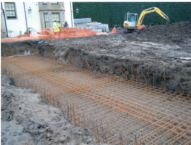
Illus 4 Area excavated to SE, with reinforcing rods in place, facing east
