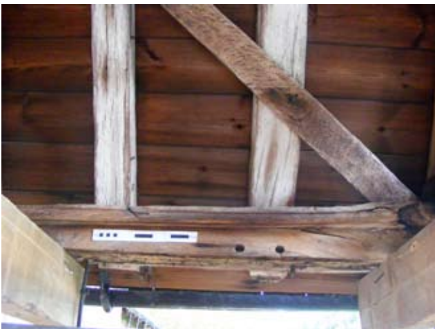
Illus 4a Close up of re-used timber in east wall plate looking E
