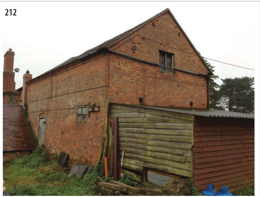
212 External view showing change in coursing for the alteration of the roof height
