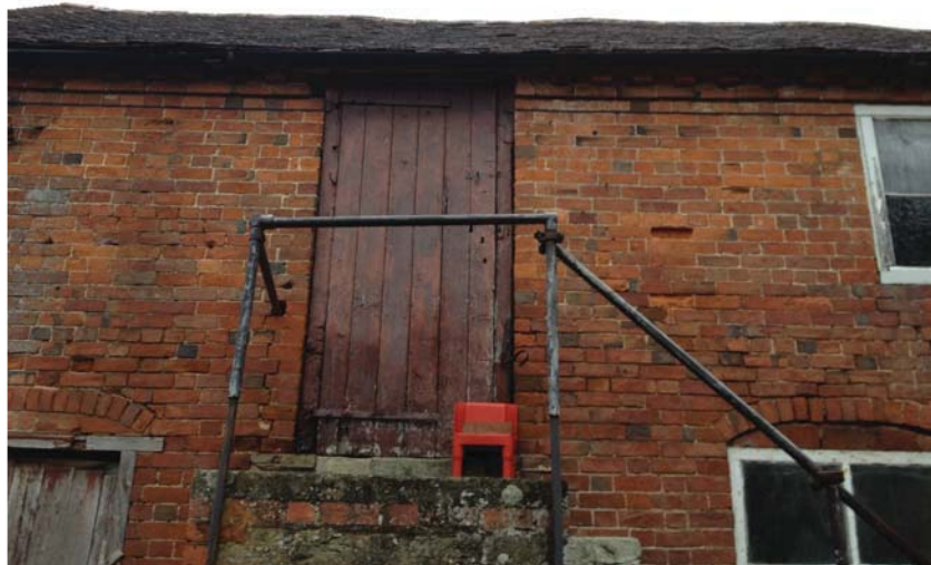
Doorway accessing upper level, due to the building constraints the lintel cuts the top of the wall below the roof level
