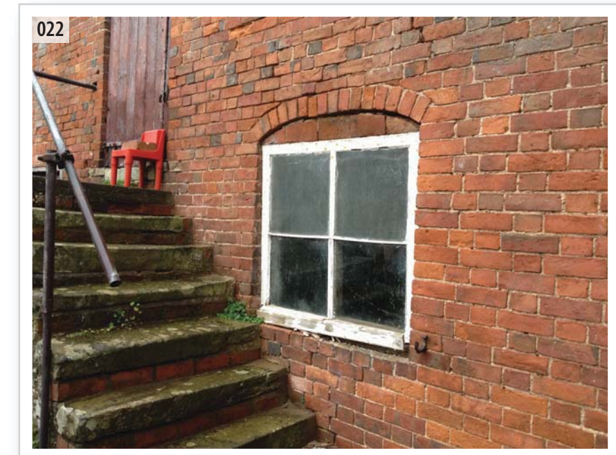
022 Arched brick lintel reflecting original lintels over inserted window, cut by later inserted staircase
