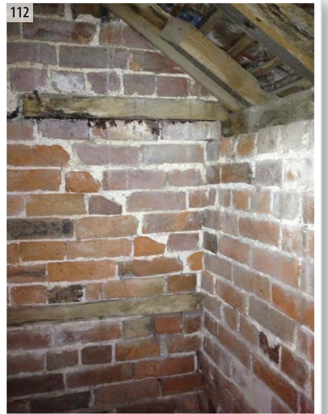
Internal view showing change in brick coursing required on the gable end because of the alteration to the roof angle and height
