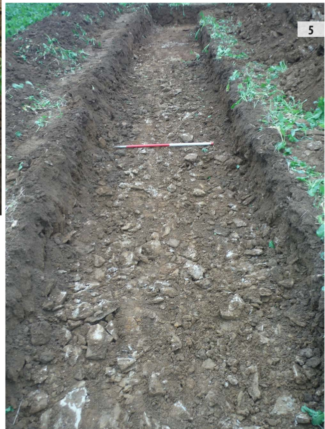
ILLUS 3 Trench 4, looking east, geological formations ILLUS 4 Excavated geological features in Trench 4 ILLUS 5 Trench 3, looking south-east, displaying high amounts of limestone brash
