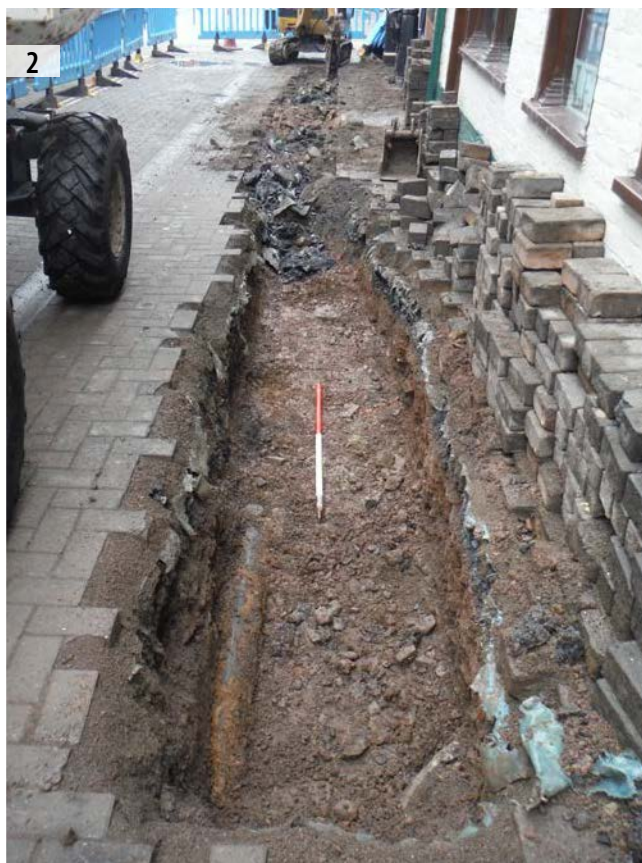
ILLUS 2 Facing west; plan shot by sample section 1 showing evidence of old pipes
