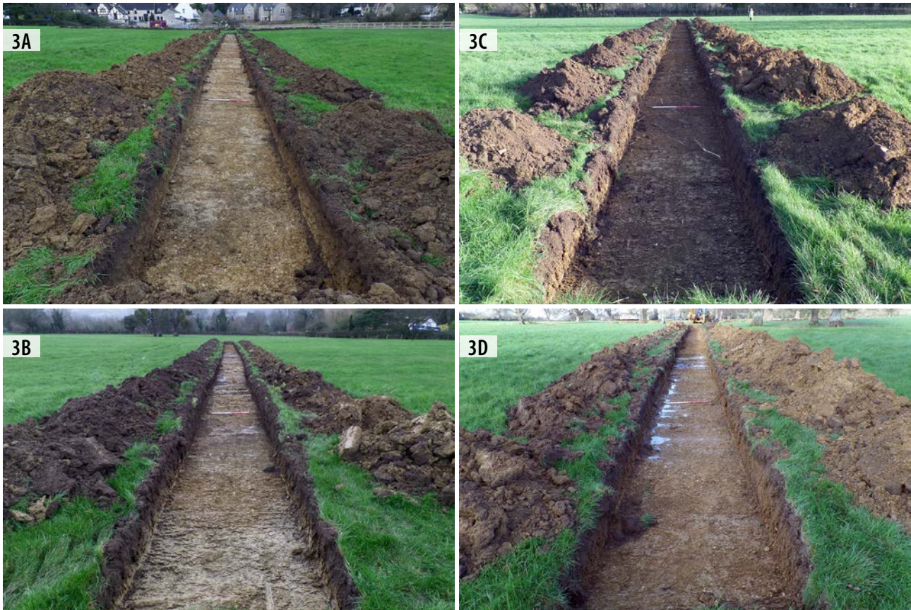
ILLUS 3A Trench 1, looking S ILLUS 3B Trench 2, looking SE ILLUS 3C Trench 3, looking E ILLUS 3D Trench 4, looking N
