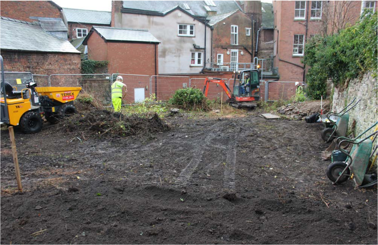
ILLUS 4 General view of site at commencement of clearing groundworks, looking north
