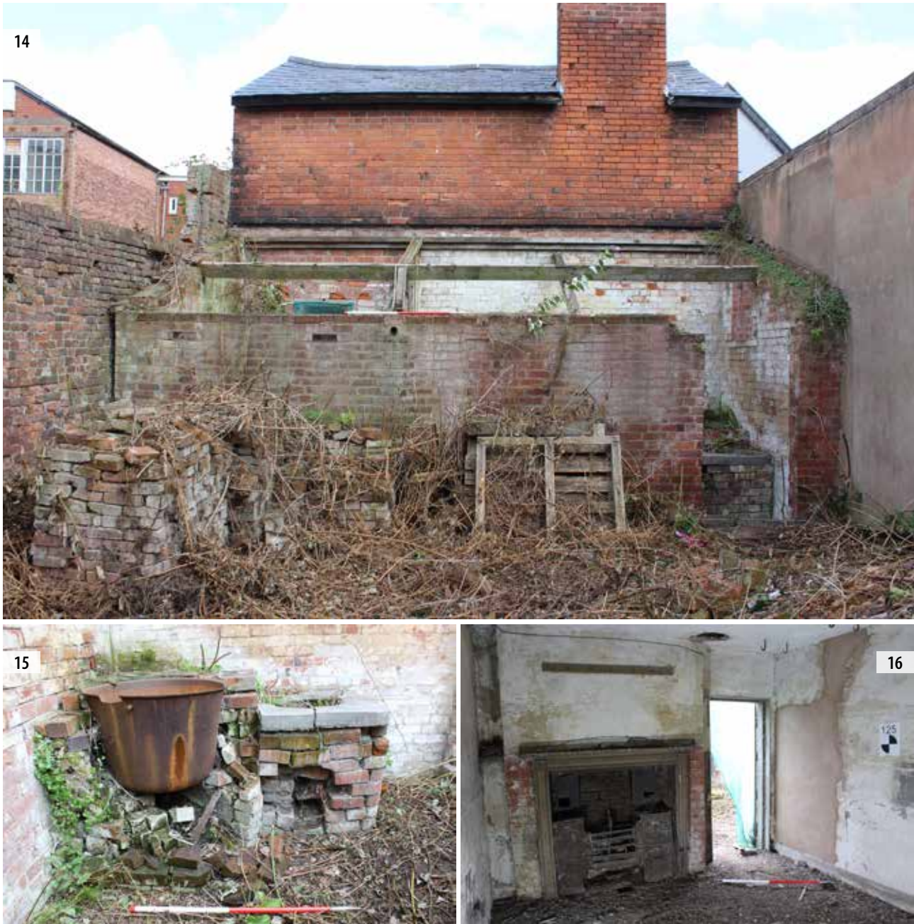
ILLUS 14 General view of Building C exterior, looking north ILLUS 15 View of copper in Building C ILLUS 16 View of interior of room 10, looking south-west
