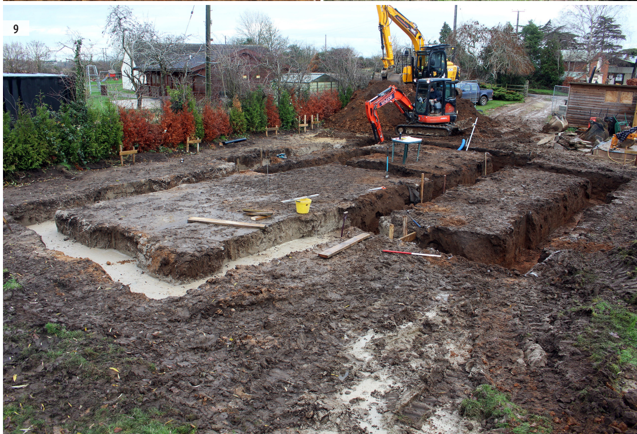
ILLUS 7 View of possible 'fire pit', looking south ILLUS 8 View of completed garage foundations looking east ILLUS 9 General view of completed house foundations, looking north-east
