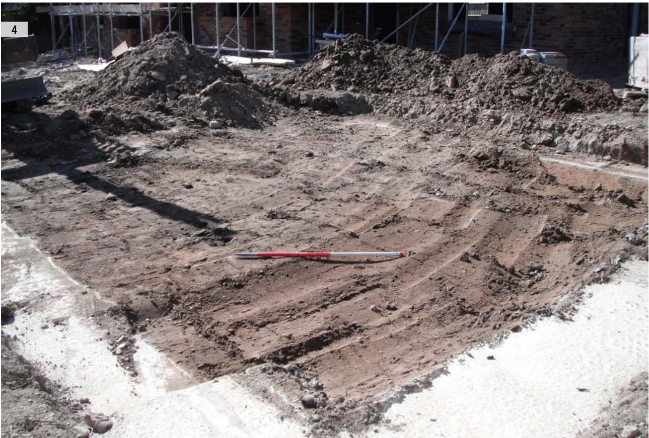
ILLUS 3 General view of road construction (topsoil strip), looking north-east ILLUS 4 General view of garage plot (topsoil strip), looking south-east
