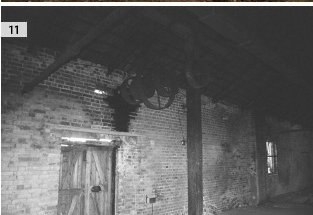
ILLUS 6 Building A exterior, northern elevation, facing south ILLUS 7 Building A interior, east-west wing, facing E ILLUS 8 Building A interior, east-west wing, lower floor ILLUS 9 Building A exterior detail – west gable, mullioned tudor window, return north-south wing visible to the right of image ILLUS 10 Building A interior detail – east-west wing lower floor, winnowing machine ILLUS 11 Building A interior detail – east-west wing, upper floor, belt-wheels
