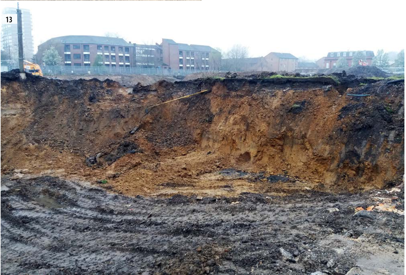
ILLUS 12 Section of pipe trench through Area 3, facing south-west ILLUS 13 Section of ground reduction in Area 4, facing north-east
