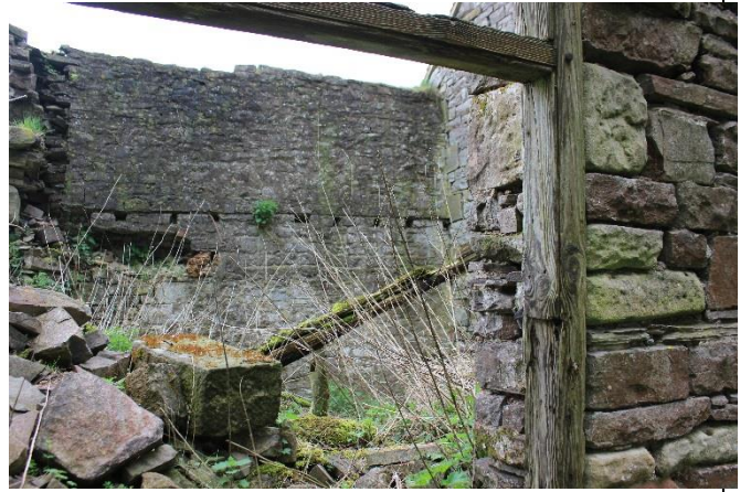
Plate 34: fallen beam and joist holes in attached outbuilding 7
