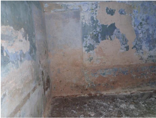
Plate 9: blocked doorways in Room 1
