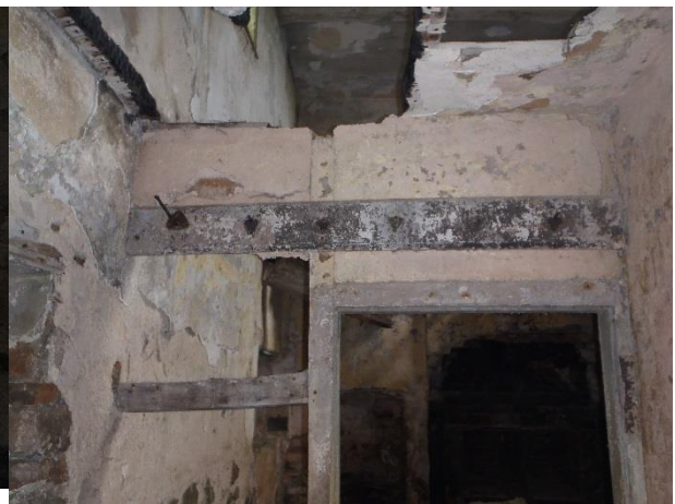
Plate 24: partition wall with coat hooks in Room 5, showing damaged ceiling
