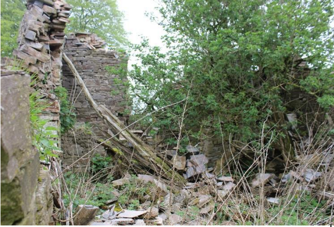
Plate 39: interior of Outbuilding B showing rubble and vegetation
