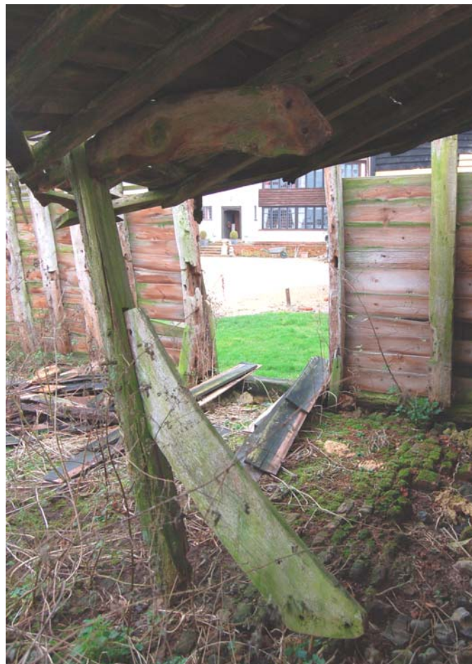
Plate 30 Collapsed south gable and remains of crown post roof
