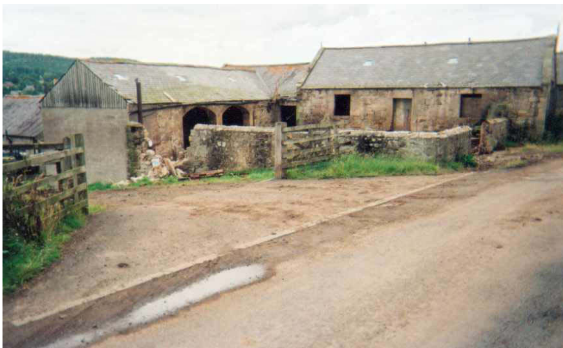
Plate 3: Rooms A and B, from the south-west, one archway is blocked on the south side of Room B
