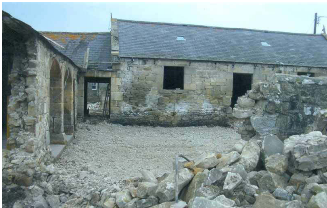
Plate 4: Room B part demolished with the through passageway visible between Rooms A and B, facing east
