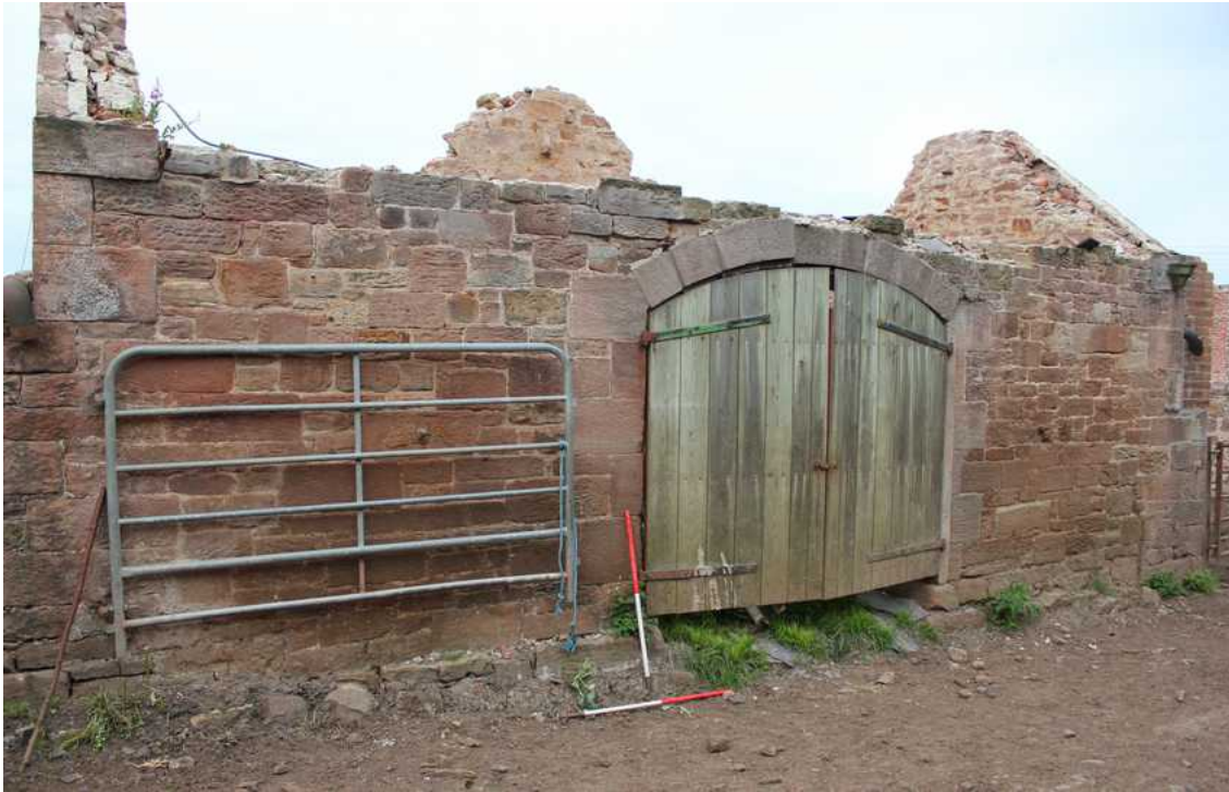
Plate 9: South face of Building D, showing double door and missing roof
