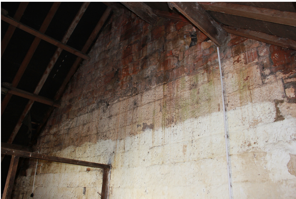
Plate 12 East wall of Room C, showing possible early roof line between large early blocks and later smaller irregularly coursed blocks
