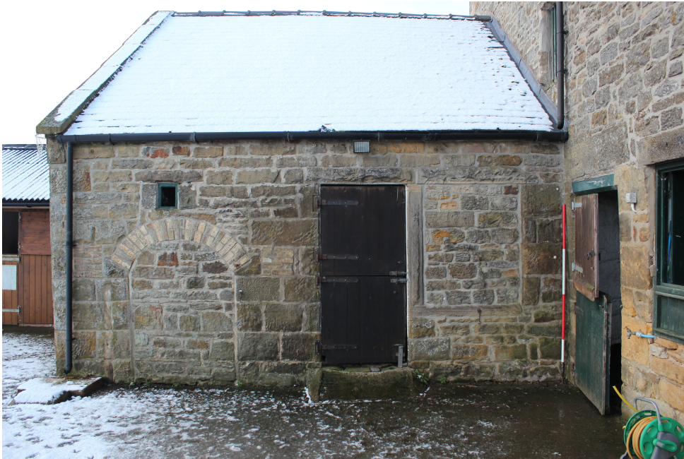
Plate 13 East wall of Room D, showing blocked arch and at least two phases of masonry
