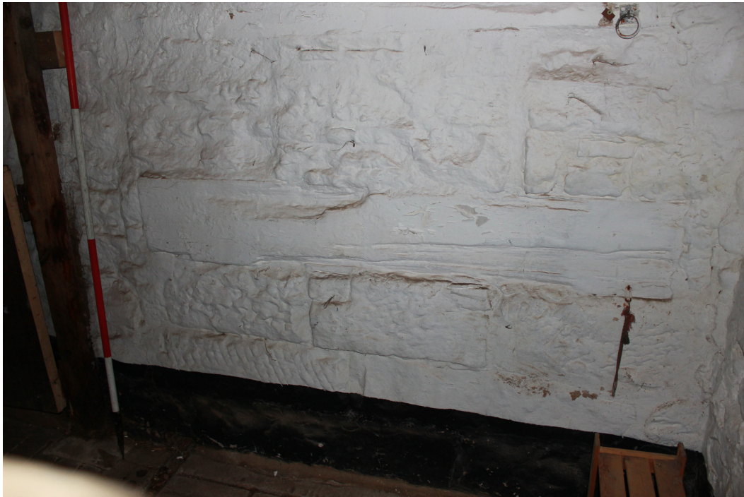
Plate 5: Large chisel tooled masonry blocks and cut timber, south-west corner of Room A
