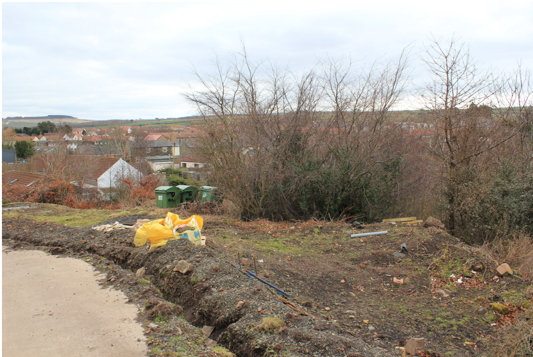
Plate 1: View of the part backfilled service trench and spoil area at the south of the proposed development, facing south west
