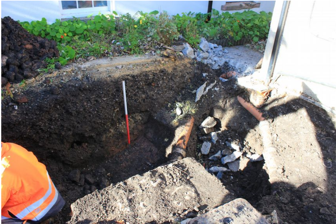
Plate 1: Excavation of the site of the new drain chamber exposed, facing north-west
