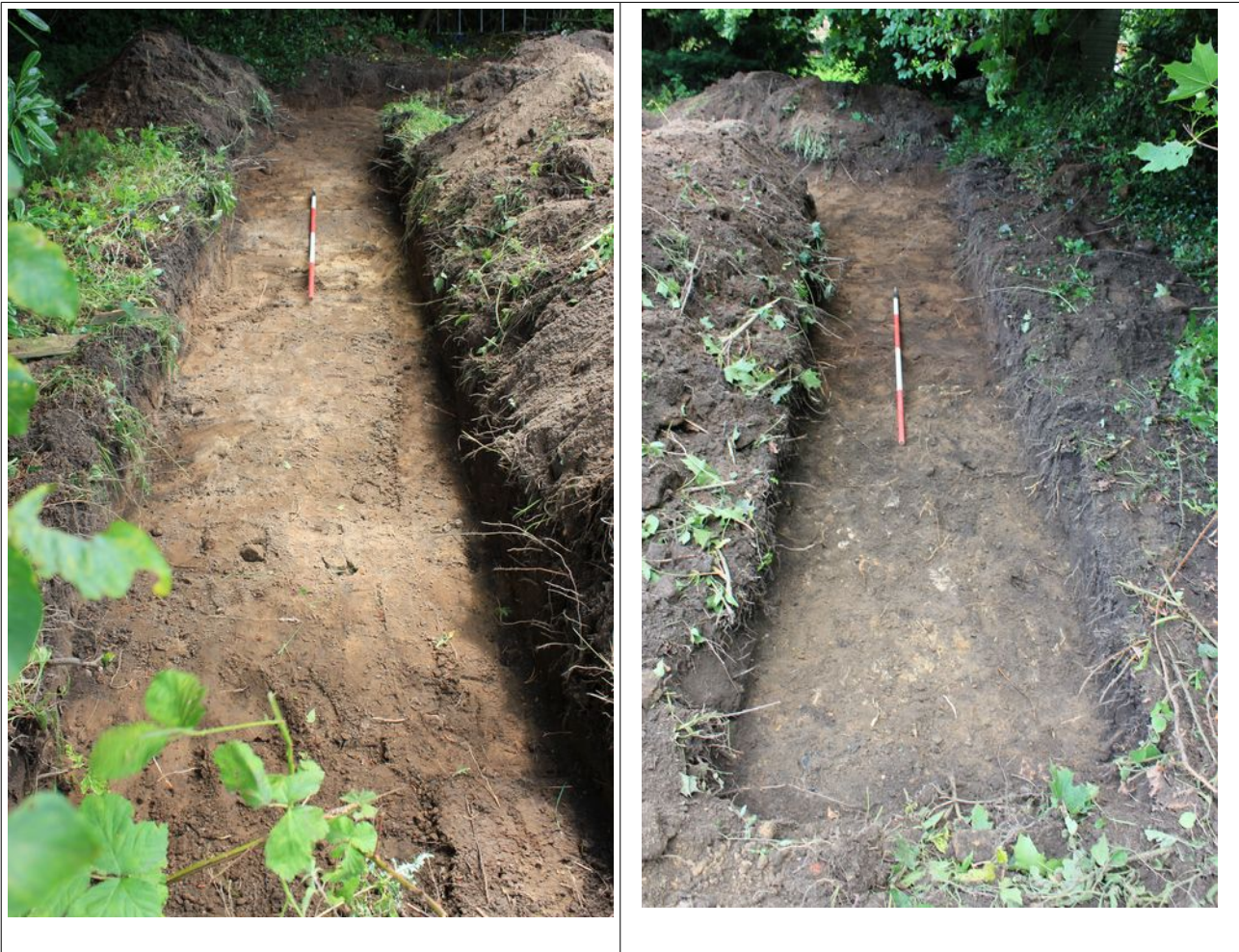
Plate 1: Trench 1, north leg on left, facing south and south leg facing east on the right
