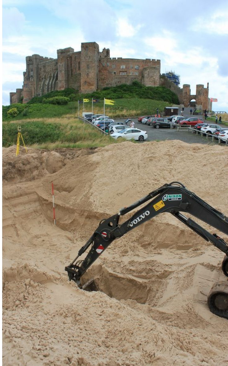
Plate 1: Deepest excavation within the trench showing the extent of the aeolian sand deposits, facing north
