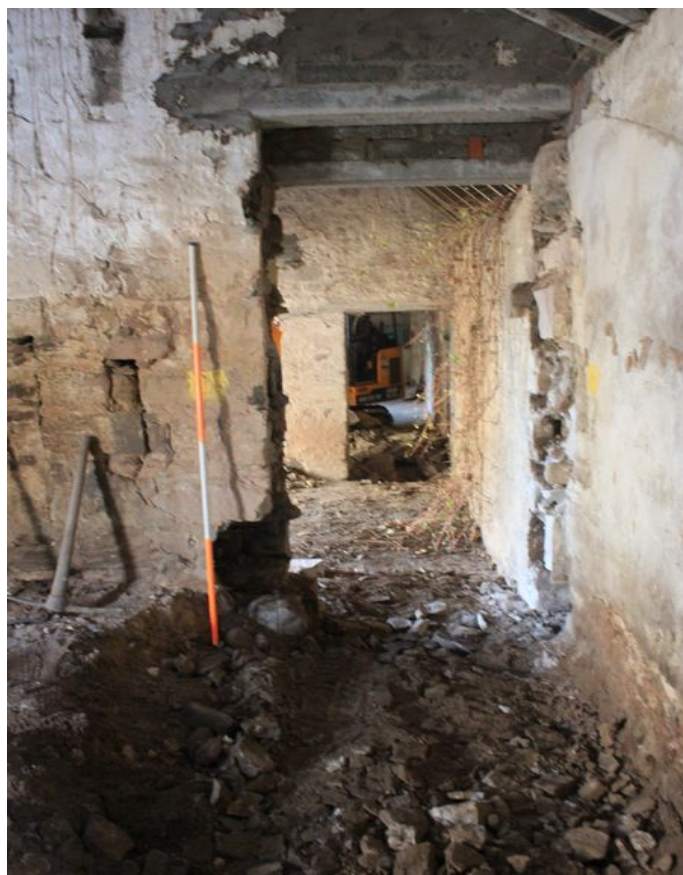
Plate 13: cut through for new doorway between Rooms B and D, facing east
