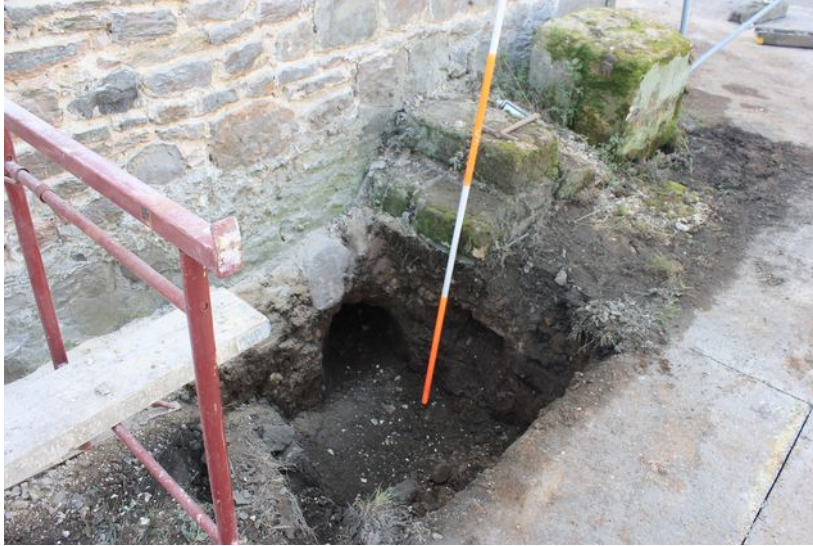
Plate 4: the stone steps at the south-west corner of the west range, facing west
