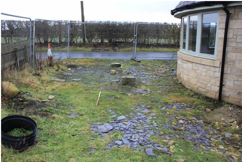
Plate 5: The site area to the west of the house at the time of the trench excavation watching brief, facing north-east
