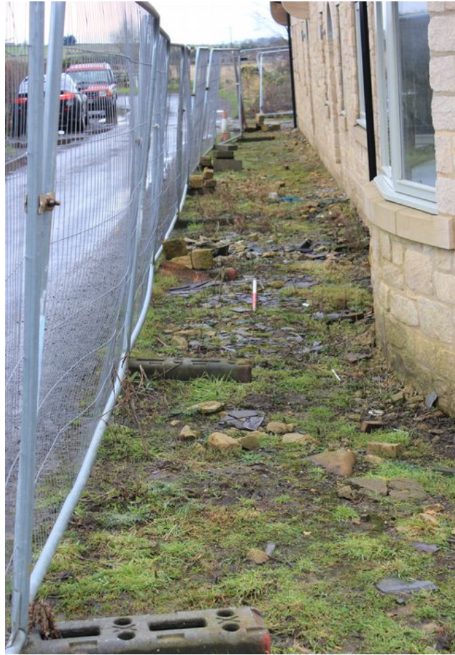
Plate 6: The area to the north of the house at the time of the trench excavation watching brief, facing east
