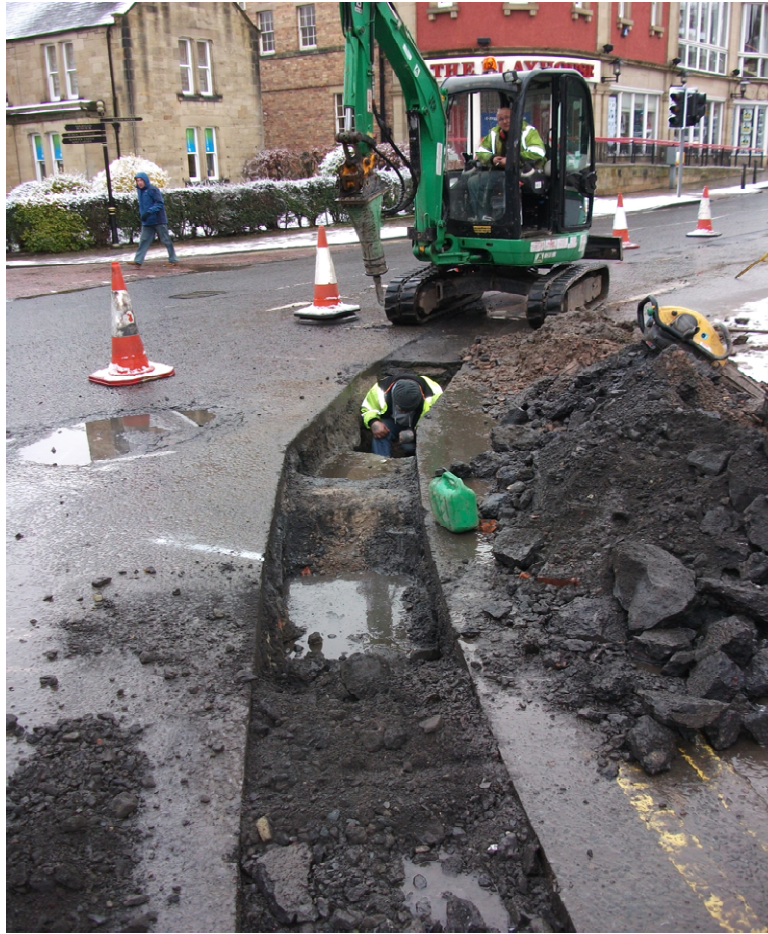
Plate 1: Installation trench at the corner of Hotspur Street with Bondgate Without, facing north east
