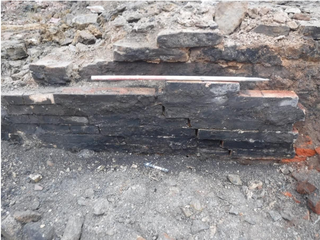
Figure 43. Photograph of poorly preserved boiler-bed wall {4008} against the background of stone wall {4010}, looking east (scale: 1x1m)
