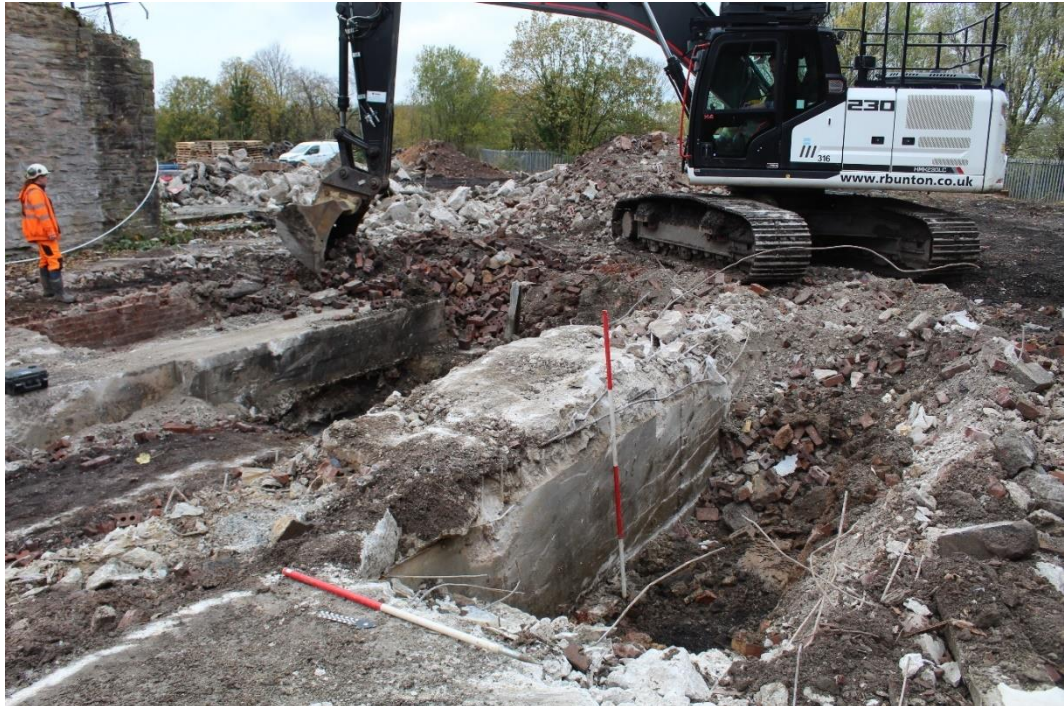
Figure 13. Working Photograph of the Area 1 excavation showing modern concrete foundations {1001} and {1003}, looking south west (scale: 1x1m, 1x2m)
