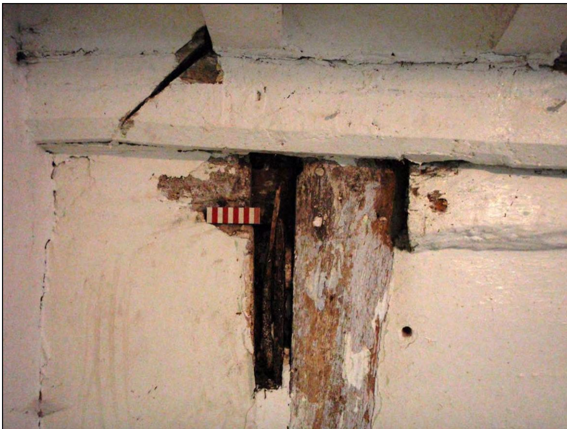
Figure 30: Detail of stud detached from rail with later cement infill, looking south (scale 100mm)
