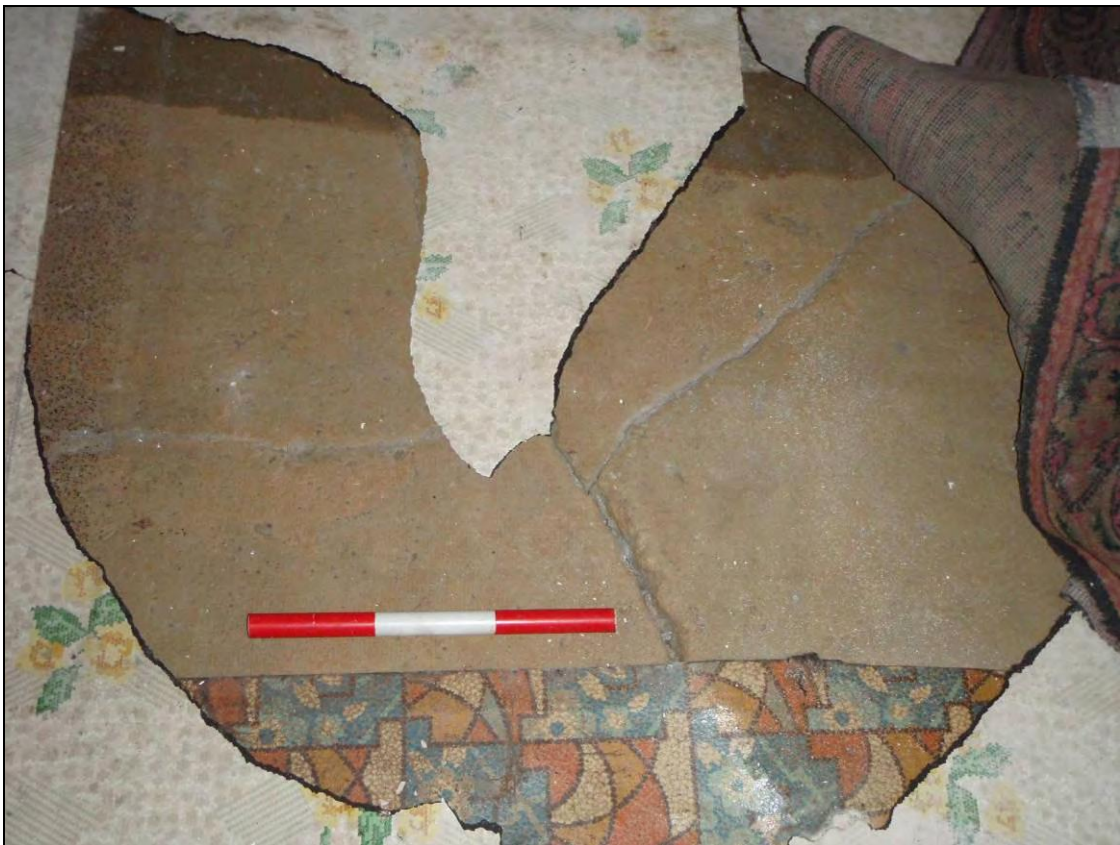
Figure 61: Fissures on the screed floor (scale 300mm)
