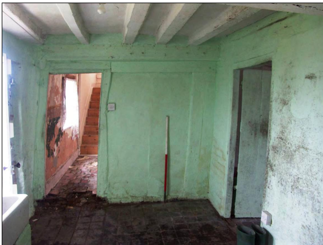
Figure 26: Eastern wall of room G-1 with surviving timber stud and rail (scale 1m)
