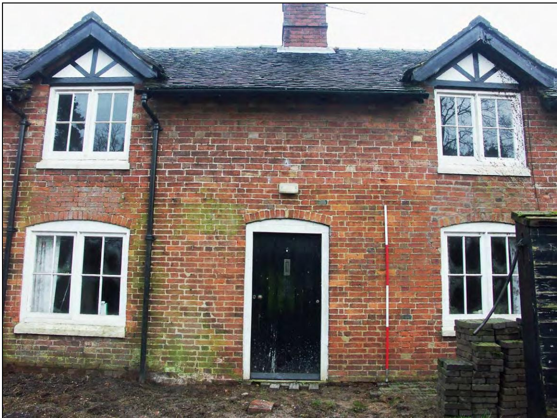
Figure 9: Doorway between the southern and central bay of the west elevation (scale 2m)
