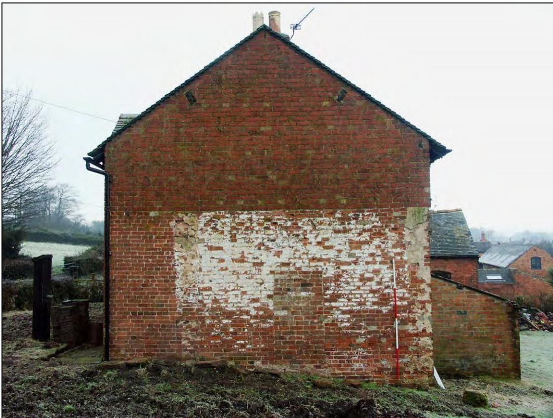
Figure 20: South elevation showing a blocked doorway and scars of a demolished structure (scale 2m)
