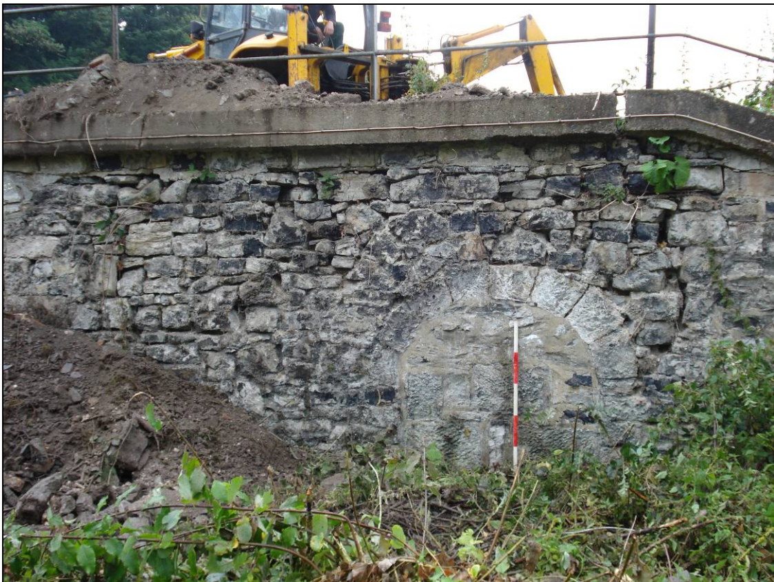
Figure 8: Arched opening of a former boiler adjacent to the stack behind the wall, looking west (scale 1m)
