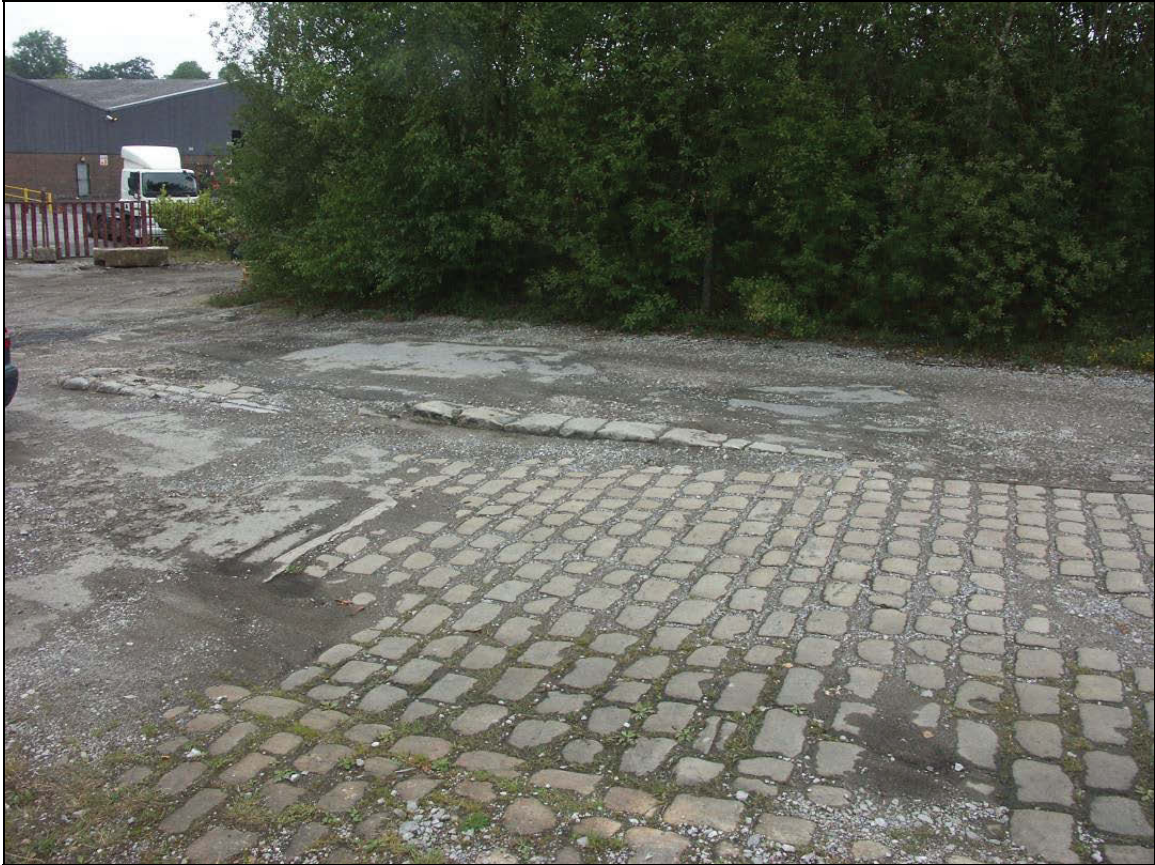
Figure 12: Viewpoint 3 –Footings of a former building adjacent to the cobbled road to the works
