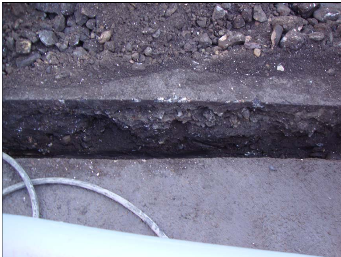
Figure 3: Section photograph of Marygate excavation, showing road make up and disturbed ground.
