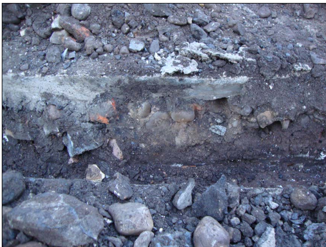
Figure 4: Section photograph of St. Cuthbert's Square excavation, showing road make up and disturbed ground.
