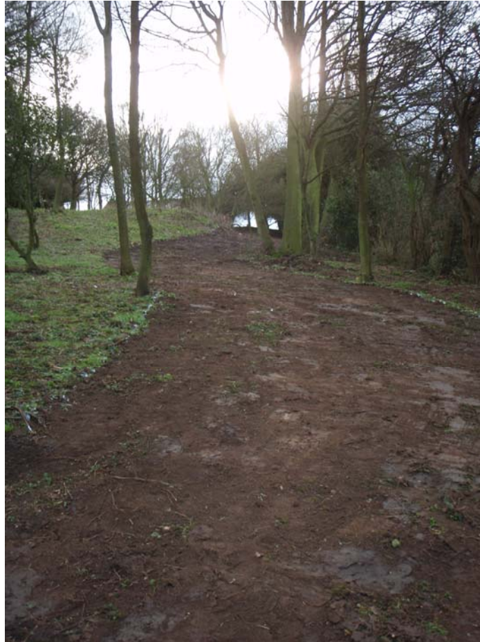
Figure 4: Stripped area through the woodland, with paler patches of natural clay showing through.
