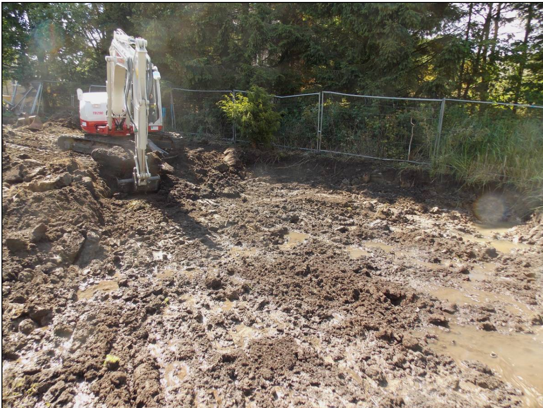
Figure 16: Plot 4 during excavation of the overburden within the northern area, looking west.
