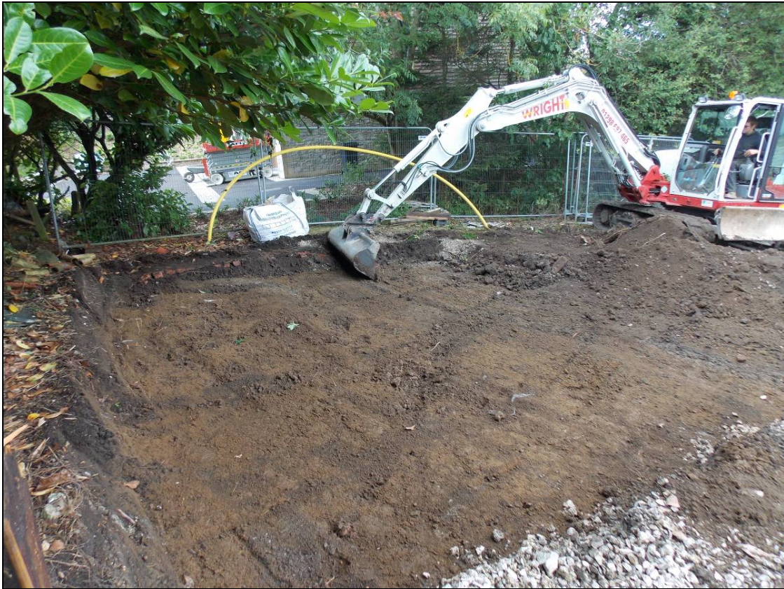
Figure 17: Plot 4 during excavation of the overburden within the southern area, looking west.
