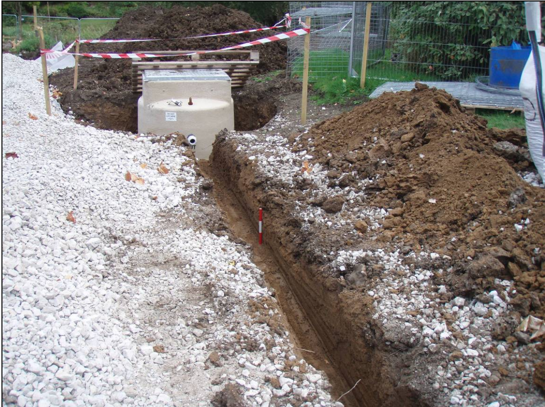
Figure 19: General view of Plot 5 with a large pit and service trenches, looking north (scale 300mm).
