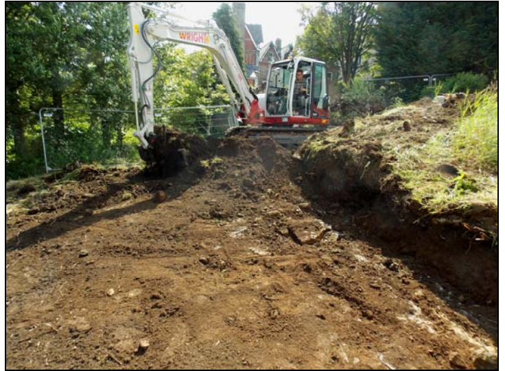
Excavation of Plot 2 with dwelling number 8 Wye Grove in the background, looking east.
