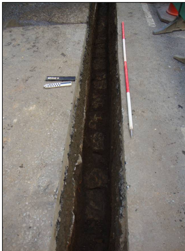
Figure 6. Section of trench showing stone lined drain running along the base of the trench. Scale = 2m.
