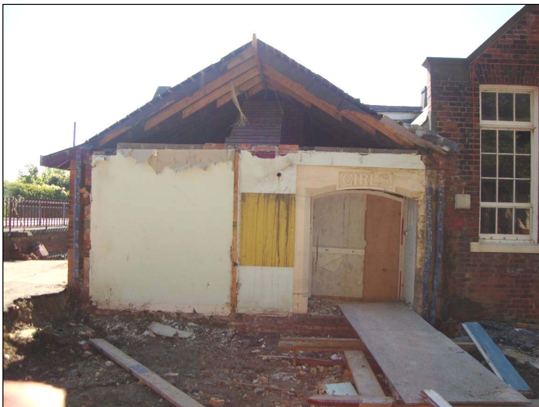
Figure 28: Northern extent of the west facing elevation showing where the extension has been demolished to reveal the original girls' entrance with inscription.
