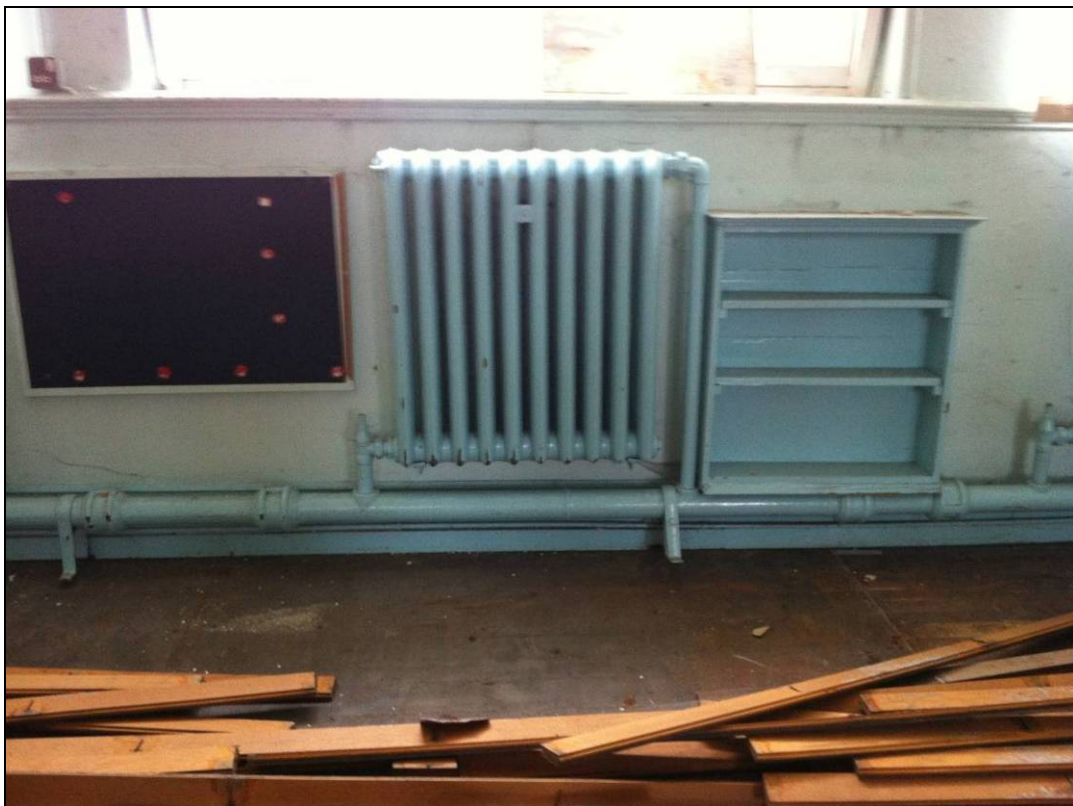
Figure 3: One of the original cast iron radiators in one of the classrooms.
