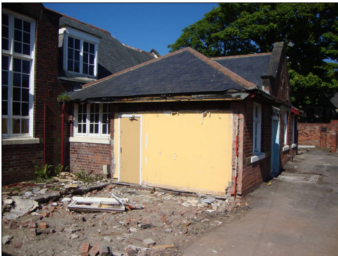
Figure 26: External east facing elevation of Room 1, looking south west and showing where the toilet block has been demolished.
