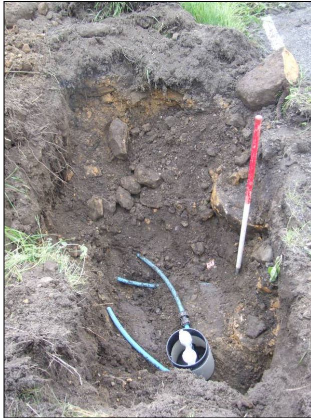
Figure 3: The southern trench showing topsoil with turf (100) and yellow sandstone rubble (101), looking west. Scale = 1m
